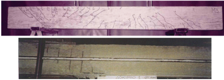
Fig. 1.18 Failure of the critical region of a simply-supported RC beam with overhang exhibiting point of contraflexure ( top ) [9], and a two-span linear RC element under the action of a constant axial force combined with cyclic lateral loading ( bottom ) [6]
