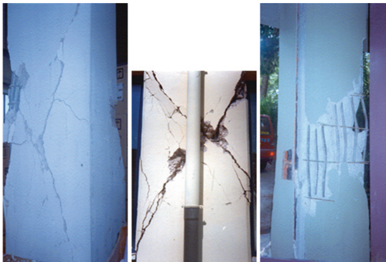
Fig. 1.19 Examples of damage suffered by columns of RC structures during the 1999 Athens earthquake [5]
