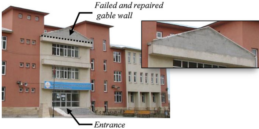
Fig. 3.1 Failed and repaired gable wall in a school building in Van (Photo taken after October 23rd, 2011 M7.2 Earthquake)
