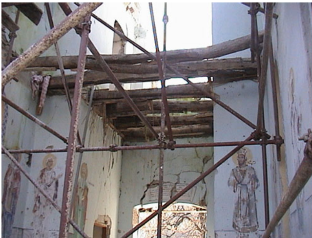
Fig. 8.14 Damage to the floor structure
