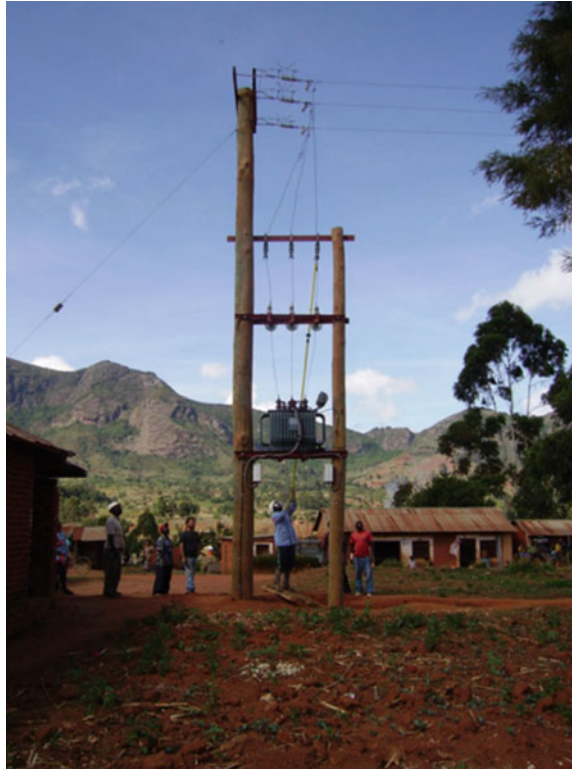
Fig. 14.2 EuropeAid (FED/2011/266-812) sustainable community based hydro-power supply in six villages of Ludewa District, Iringa Region (ACRA)
