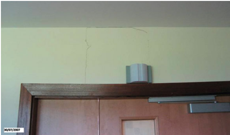
Fig. 15 Top of door binding against architrave
