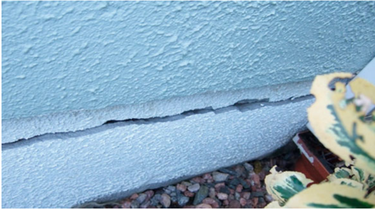
Fig. 18 Cracking and displacement of external wall (plinth)
