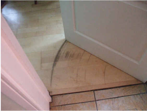
Fig. 14 Bottom of door binding against floor
