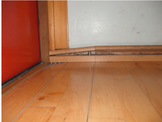
Fig. 12 Displacement of timber skirting
