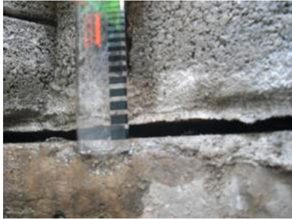
Fig. 22 12 mm gap near top of manhole
