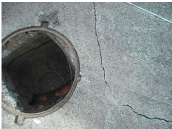
Fig. 21 Pavement cracking near manhole
