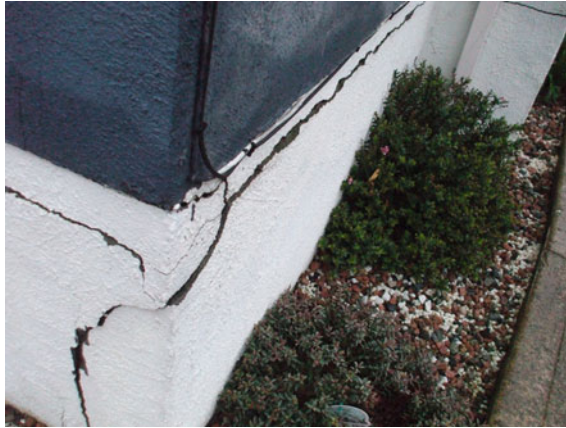
Fig. 5 Cracks created during lateral displacement of a rising wall
