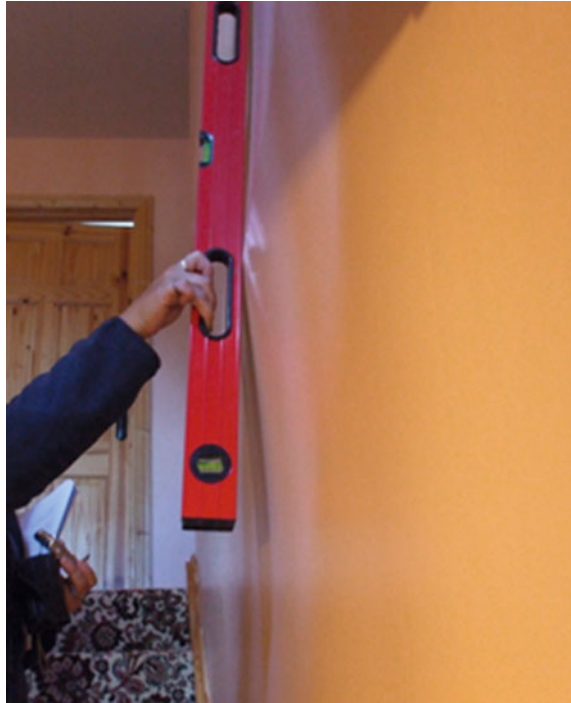
Fig. 11 Bowing of a stud wall pushed upwards by the rising floor slab
