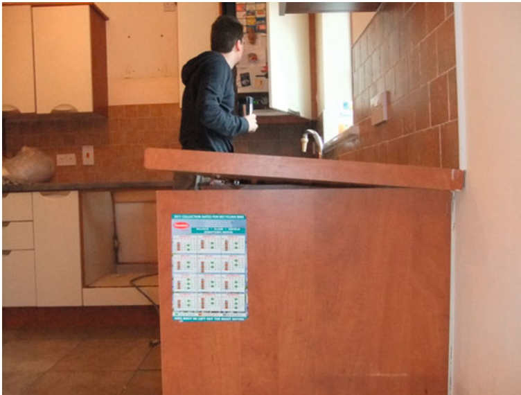
Fig. 13 Kitchen work top prised off its base
