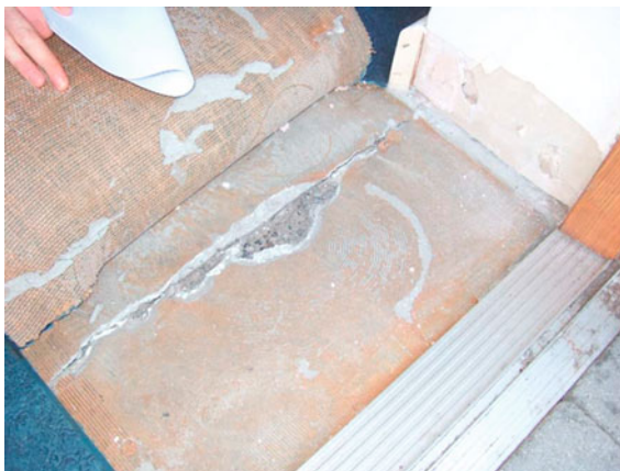
Fig. 17 Rise of floor against the threshold into the stairwell (November 2007)
