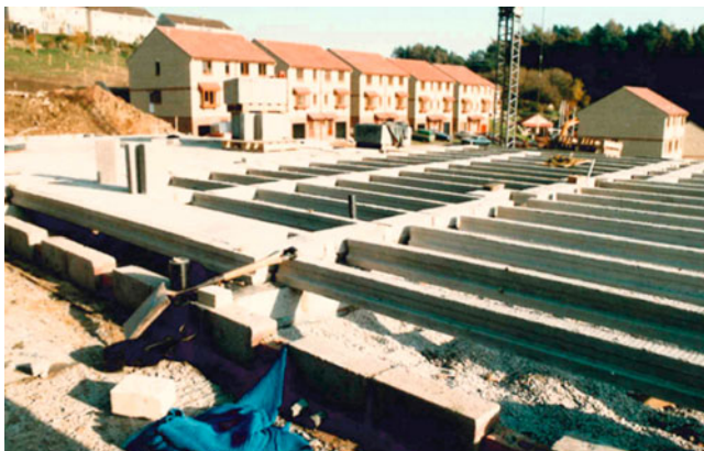
Fig. 45 Suspended floor slabs recommended for houses constructed over pyrite-rich Westbury Beds at Radstock, N Somerset
