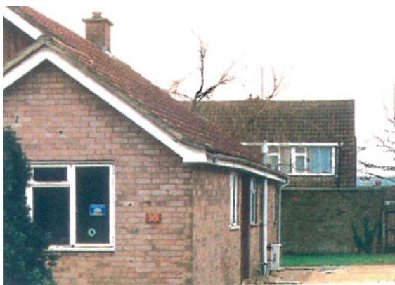
Fig. 51 Significant arch in front facade of the same bungalow as in Fig. 50
