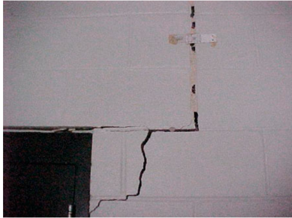
Fig. 25 Large cracks (1 inch) in concrete block adjacent to doorway. Note the attempt to bracket the wall cracks
