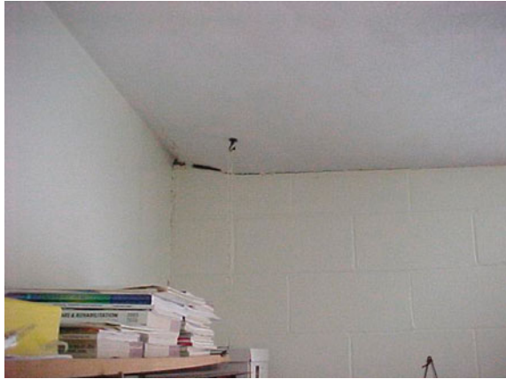
Fig. 27 Displacement of ceiling wall-board along non-load bearing walls due to floor heaving
