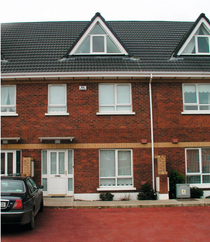
Fig. 3 The second reported house in Ireland with pyrite-induced floor heave, Dublin
