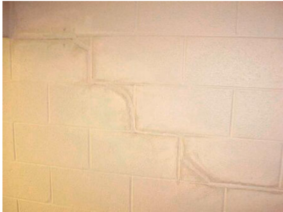
Fig. 13 Repaired masonry block cracks
