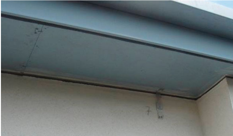
Fig. 20 Gap of some 40 mm which developed at eaves level within 5 years of construction
