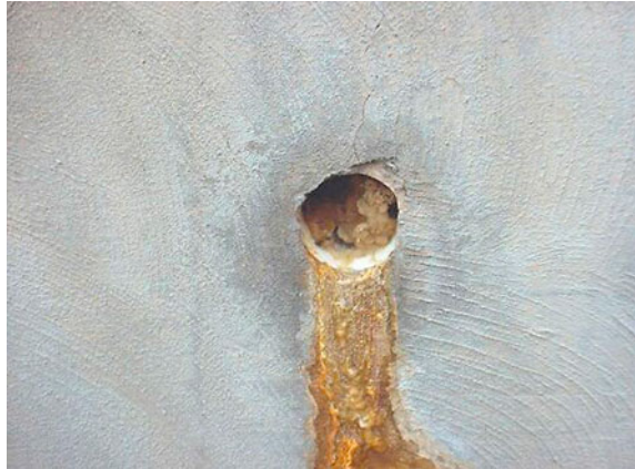
Fig. 20 Sulphate precipitates around drain pipe (2000)
