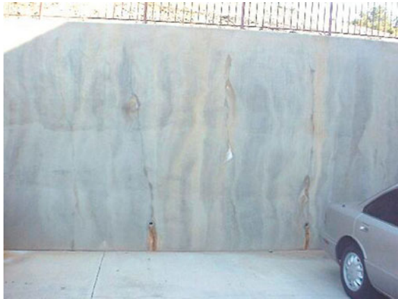
Fig. 19 Tension fractures in retaining wall; note iron stained drain holes (2000)
