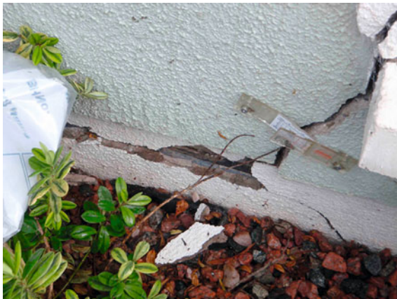
Fig. 1 Horizontal and vertical displacement due to pyritic heave in a domestic property in the Dublin area. The vertical displacement is of the order of 5–7 mm and the horizontal displacement is in excess of 10 mm
