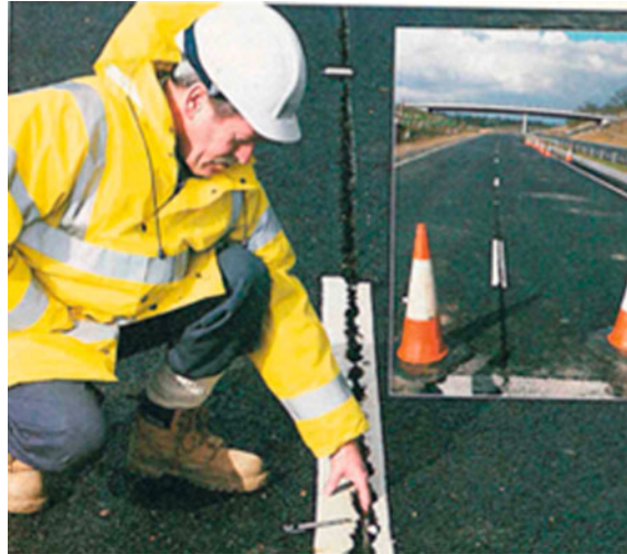
Fig. 55 Distress in the A10 (north of London) following lime stabilisation of sulphate-rich soils (New Civil Engineer 25 March 2004)
