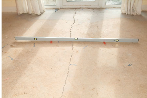
Fig. 9 Crack up to 7 mm wide across a floor which has risen 30 mm within a distance of 2.5 m
