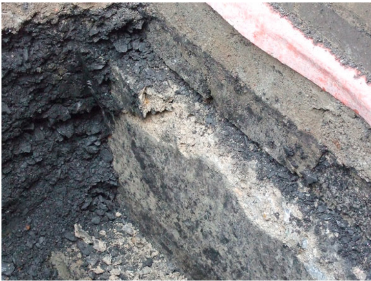
Fig. 28 Deterioration of concrete at the top of the beam, TP 11, and the nature of the dark deleterious fill adjacent to it
