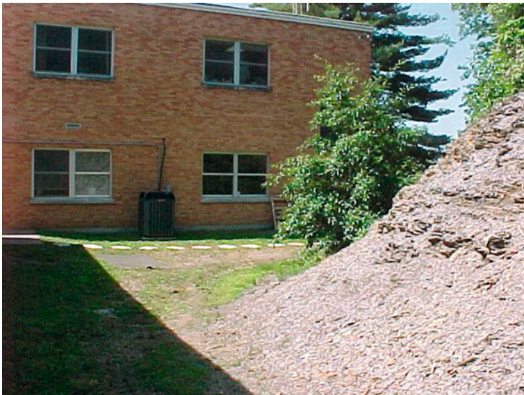
Fig. 26 Exterior of the Marcum and Wallace Hospital office wing and an adjacent outcrop of the Cleveland Member of the Chattanooga (Ohio) Shale. Note the absence of cracks or offsets in the load bearing walls and exterior brickwork of rooms with heaved floor slabs
