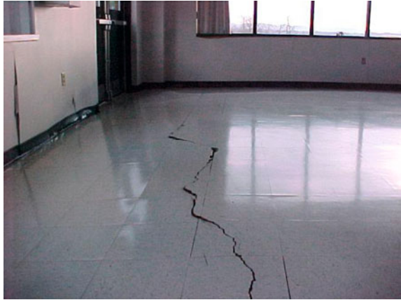
Fig. 22 Substantial floor cracks in Carhartt break room; rise of walls has caused the window to be inoperable
