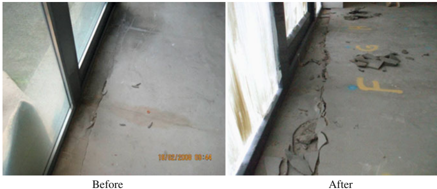
Fig. 6 Effect on the ground-bearing floor slab after the removal of fill in an adjacent property
