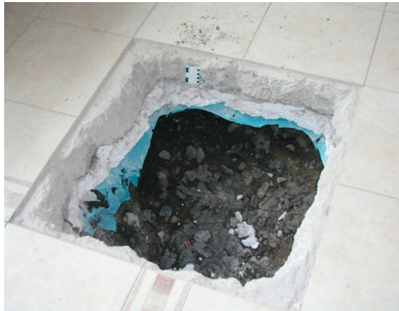
Fig. 4 Trial pit through kitchen floor exposing problematic underfloor fill
