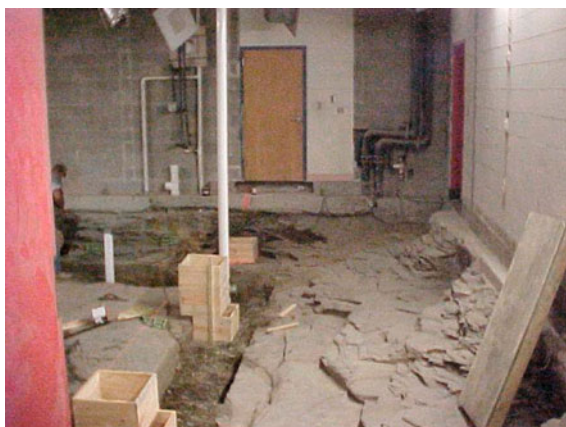
Fig. 16 Shale beneath School and new trench construction for column footers, new and old sewer PVC pipe, cleats with the sulphate mineral
