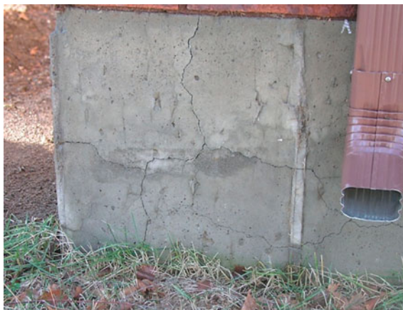
Fig. 20 Typical damage in exposed house concrete, Trois-Rivières, Québec
