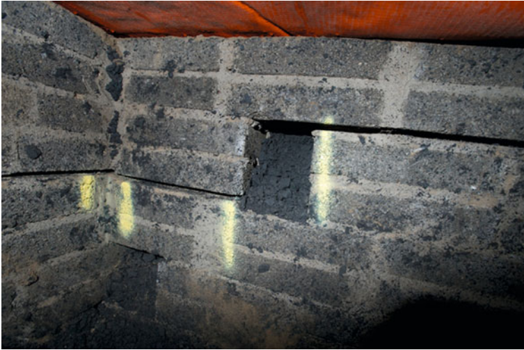
Fig. 7 Horizontal gaps (up to 20 mm) observed in a rising wall immediately after the fill was removed in a localised trial pit (the balance of the fill beneath the floor slab was still in place at this time)
