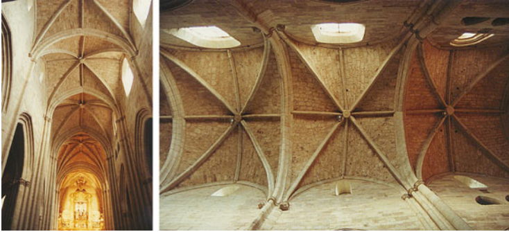
Fig. 22.1 Main nave of the Church of Santa Maria la Real, Najera, Spain. A geometric analysis of the church shows the vaulting system to be completely distorted. Arches and vaults are deformed, the walls and columns are bent, and cracks appear in the aisles. Geometry is the first test to verify the structural state of a Gothic construction. Photos: authors
