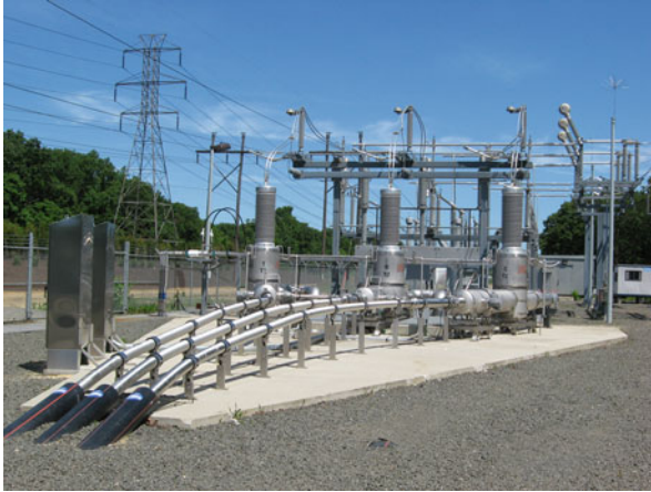
Fig. 27.20 LIPA HTS cable project (Courtesy of AMSC)
