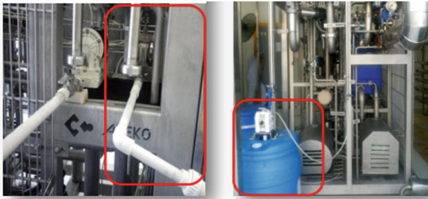
Fig. 6. Relocation of the soda dosing pump, to facilitate intervention, cleaning and maintenance tasks.
