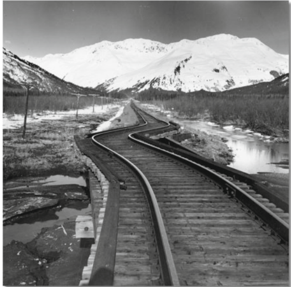
Fig. 4.6 Twisted rails near Whittier as a result earth movements during the Alaska earthquake of 1964 [4]
