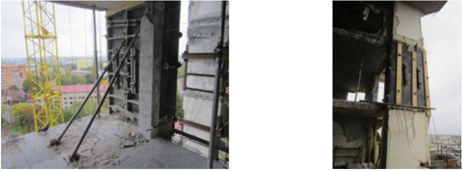
Fig. 2. Pylon in the formwork during the second stage of work. (Photo Oleh Tabarkevych).
