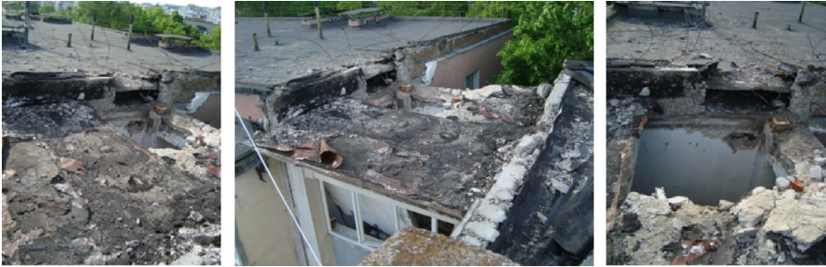
Fig. 1. Nataliia Tabarkevych. The consequences of a shell fragment hitting the floor slab of a residential building.
