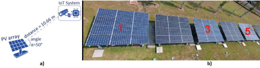
Fig. 1. a) Location of the fault detection system camera with respect to the PV array under analysis. b) PV installation used for the research. Arrays 1, 3 and 5 are polycrystalline of 12 modules each
