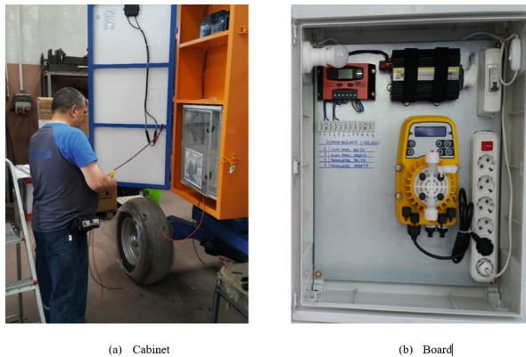
Fig. 5. Images of cabinet and board
