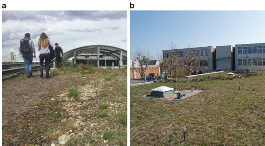
Fig. 8.6 Biodiversity key design features: (a) varying substrate thickness and type on the biodiverse green roof of the Jacob Burckhardt Haus in Basel (Author's photo); (b) woodpiles on the biodiverse green roof of the Primarstufe (Kindergarten und Primarschule) in Muttenz (Author's photo)
