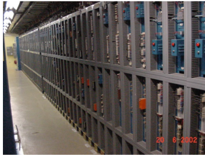
Fig. 1. A bay in the electrical room of a 900MW PWR power plant
