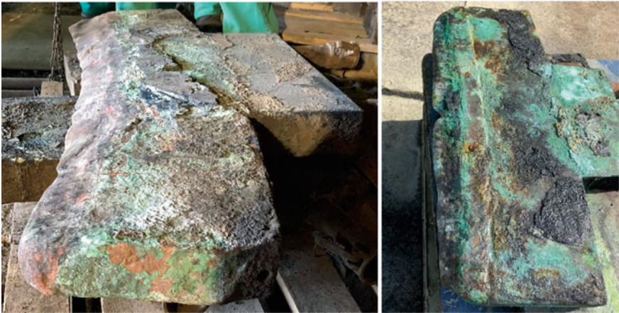
Fig. 1 Examples of corroded copper plate coolers removed from Sibanye-Stillwater Furnace 2
