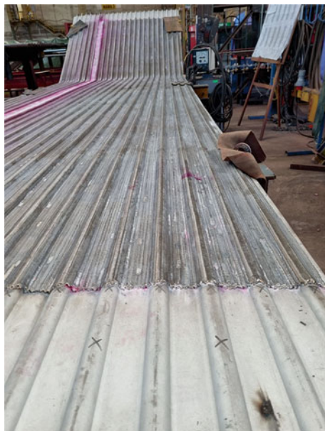
Fig. 13 Fin tube boiler wall with overlay welding
