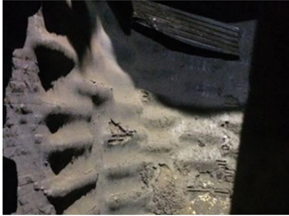
Fig. 4 Worn refractory wall with horizontal plate coolers to arrest wear [1]
