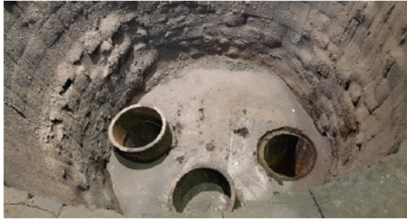
Fig. 8 Standard magnesia-chromite bricks installed above the left leg and magnesia-chromite with the Flexosphere technology installed above the right leg in the RH vessel
