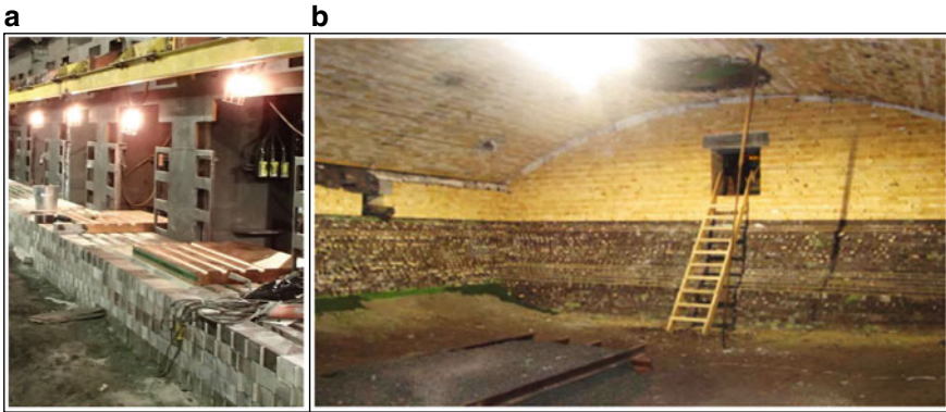
Fig. 3 a 2004 rebuild—upgrade to drilled Cu plate coolers. View along north wall. b 2004 rebuild—roof and matte endwall completed
