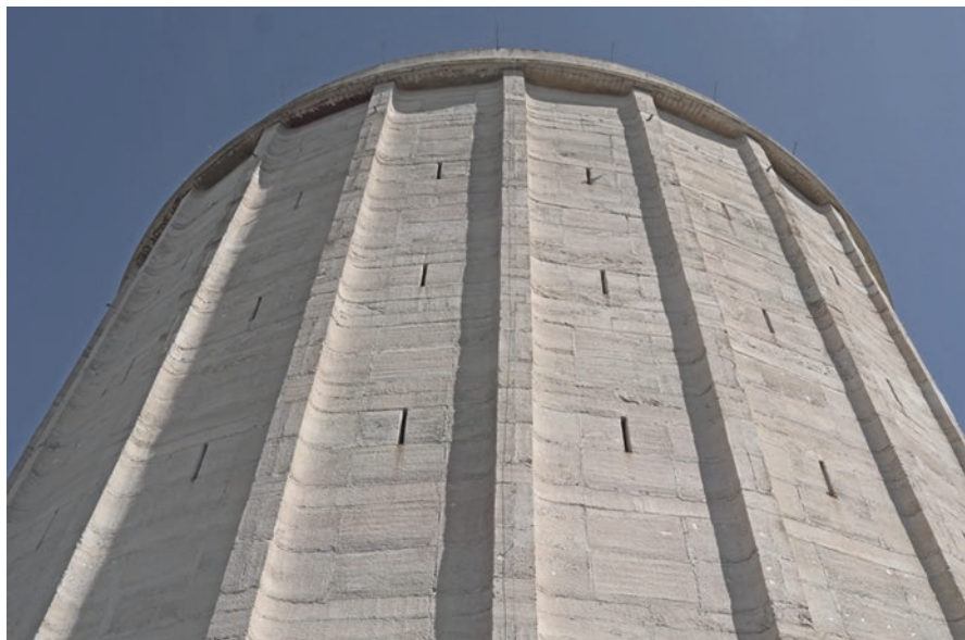
Fig. 16.10 External masonry wall of the Water Tank, with prefabricated concrete blocks in rows and cast-in-place concrete curbs. (© Vitangelo Ardito 2023)
