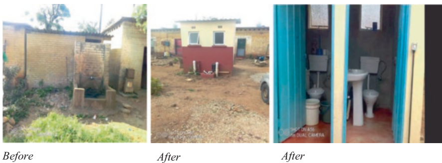
Fig. 15.5 Pre- and post-refurbishment of facilities. (Source: Inclusive Urban Infrastructure Fieldwork: Young Community Contacts (2022))
