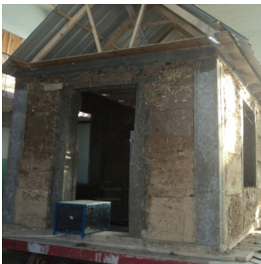
Fig. 5 The process of construction of model homes from the «reinforced concrete frame»
