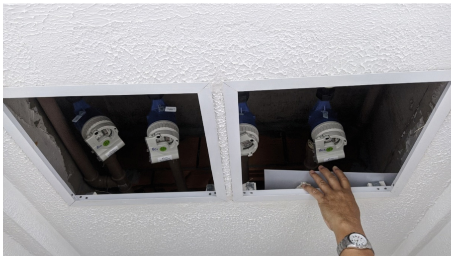
Fig. 3. Inspection boxes of the water meters located on the ceiling of the common areas between the floors. Source: Author's Collection, 2021.
