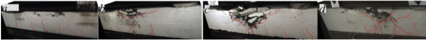
Fig. 11 The pattern of crack development at the moment of reaching the maximum displacements of reinforced concrete beams BDTY-11 (a), BDTYe-12 (b), BDTYe-13 (c), BDTYe-14 (g) under short-term dynamic loading
