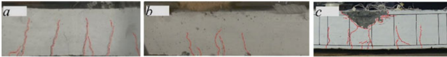
Fig. 7 Pattern of crack development at the moment of reaching maximum displacements of reinforced concrete beams BD-3 (a), BDT-4 (b), BDT-5 (c) on rigid supports under short-term dynamic loading
