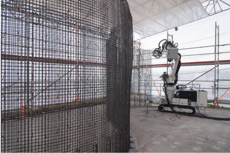
Fig. 1 The in situ fabricator building the mesh mould at the NEST house. The mesh mould process unifies the reinforcement and formwork production into a single and robotically controlled on-site fabrication system. (Image courtesy: NCCR Digital Fabrication)
