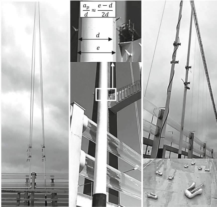
Fig. 1 RWIV and VIV of longest hangers (left and middle) wind normal to the hanger plane. Overlay of two video frames at the extreme excursions of the cable. Failed stockbridge dampers displaying empty clamps and damper masses scattered on the bridge deck (right)
