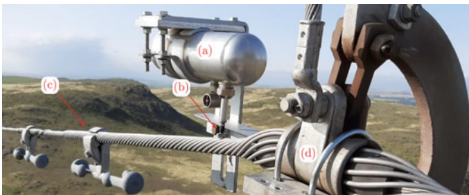
Fig. 3 VIBREC 500 installation detail (a) VIBREC 500 sensor, (b) Input arm of the recorder, (c) OPGW cable and Stockbridge damper system, and (d) Suspension clamp
