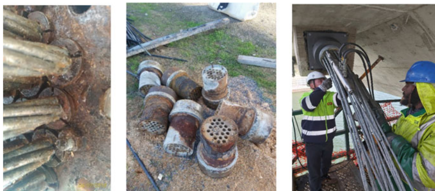
Fig. 2 During inspection water leakage at deck anchorages was found (left); Deck anchorages after removal (middle); Installation of new stay cables with ConTen system (right)
