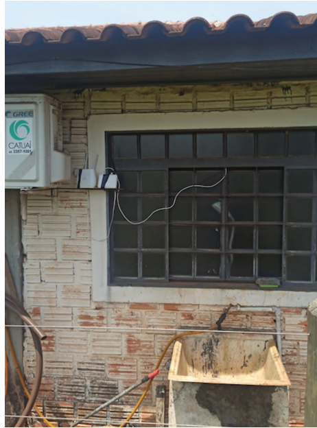
Fig. 8. Gateway installed on the farm. No need of complex infrastructures.
