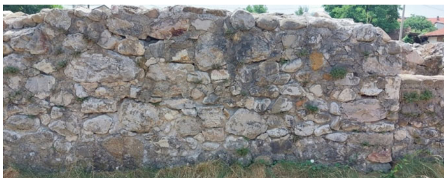
Fig. 4 Weeds grew from south wall joints on June 29th, 2022 ( Source Photo is taken by Authors)
