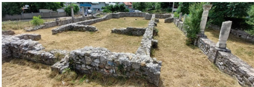
Fig. 3 Bushy vegetation is deteriorating stone walls on June 29th, 2022 ( Source Photo is taken by Authors)
