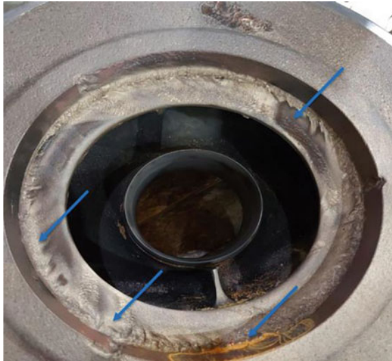
Fig. 7 A loose and wear of the casing wear ring of 1st impeller
