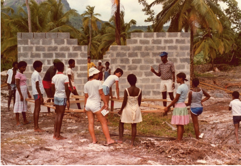
Image 27.3 A work crew of students and animateurs (youth leaders) prepare to raise a roof truss in a classroom. (Image: Hubert Murray, 1981)
