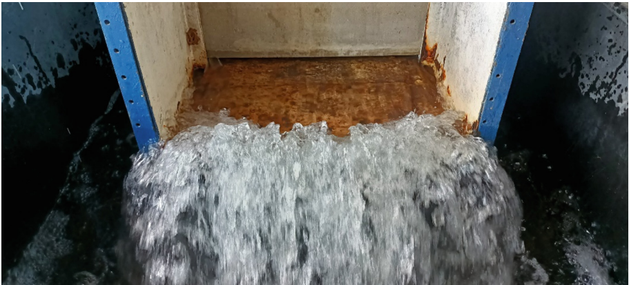
Fig. 4. Outlet condition of Gate Partially Open with opening 2cm.
