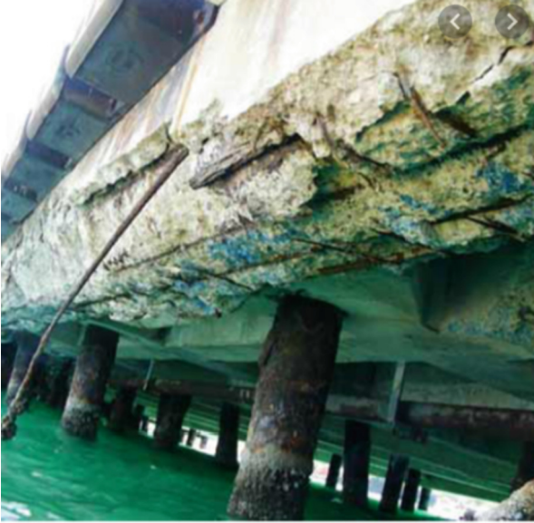
Fig. 7. The condition of deteriorated structure after sulphate and chloride attack.
