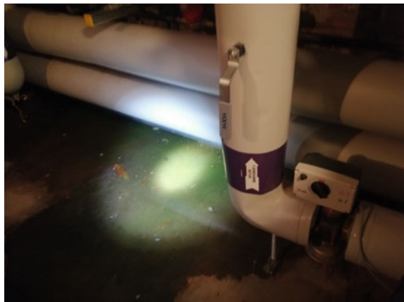
Fig. 2 Green water of district heating (chemically altered by the utility company to be distinguishable from drinking water when leaking from pipes) in the basement of an apartment building in Denmark
