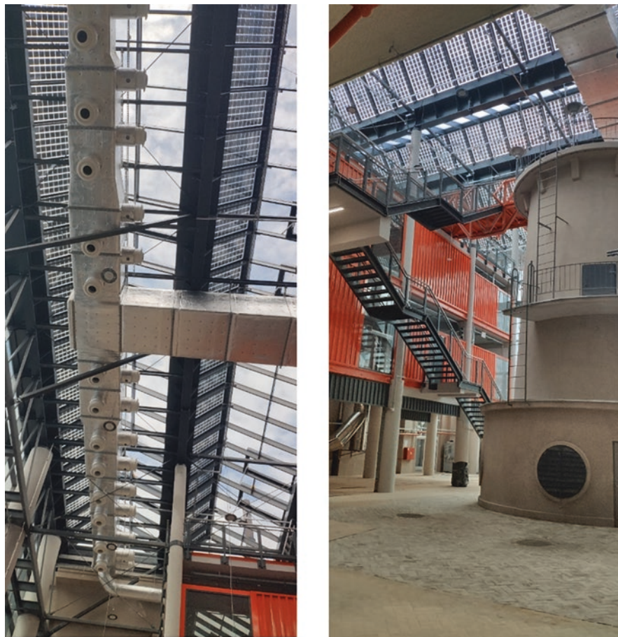
Fig. 14 BIPV system in a form of glass-to-glass technology
