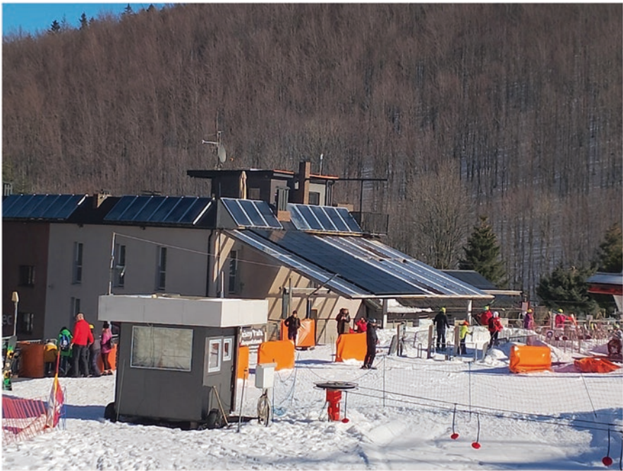
Fig. 7 New photovoltaic installations next to the previously installed solar thermal collectors on a building of the ski lift center
