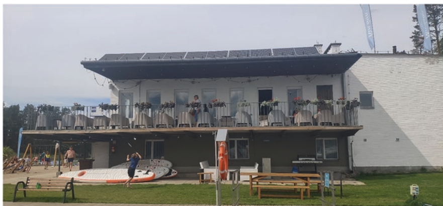
Fig. 10 PV modules placed on horizontal roof on support constructions
