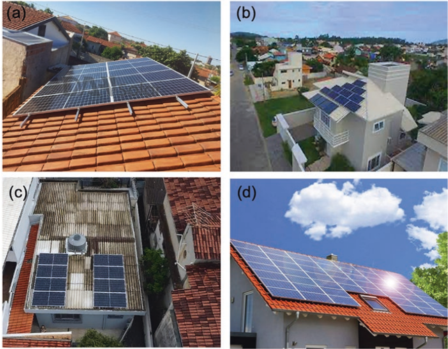
Fig. 19 Examples of BAPV in Brazil: (a) 4-kW on red tile roof; (b) 3 KW on cement roof; (c) 4 kW on galvanized steel roof; and (d) 6 kW on tile roof
