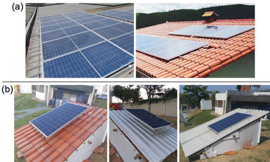
Fig. 25 (a) Two PV roof installations in Minas Gerais (formed part of survey); and (b) Installations for determining the optimum module-roof separation for 3 common roofing materials in Belo Horizonte, Brazil. Left to right: Red-ceramic tile; galvanized steel, cement (based upon the report of Guimaraes [73])
