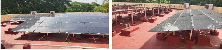
Fig. 13 Solar PV installation on the terrace
