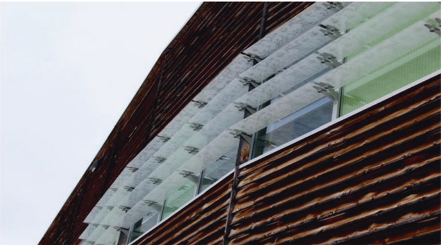
Fig. 28 Mounted solar shading louvers on a window of the Vale Living with Lakes Centres, Greater Sudbury – Ontario, Canada. (Image credit and source: Student3132021, https://commons.m.wikimedia.org/wiki/File:Exterior_solar_shading_fins_on_the_Vale_Living_with_Lakes_Centre.jpg )
