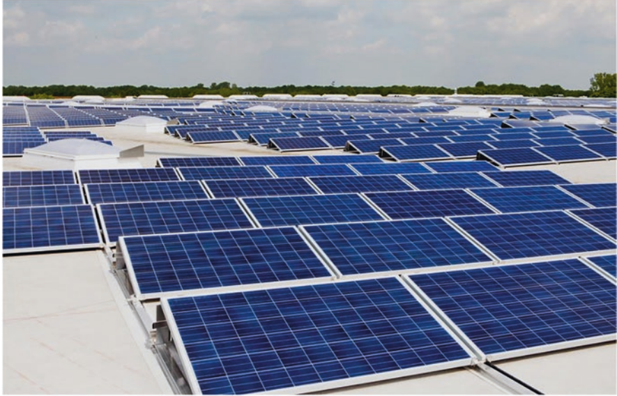
Fig. 15 A large integrated PV on the rooftop of Hannover building generating 1 MW power. (Image credit and source: AleSpa, https://upload.wikimedia.org/wikipedia/commons/b/b8/Photovoltaik_Dachanlage_Hannover_-_Schwarze_Heide_-_1_MW.jpg )
