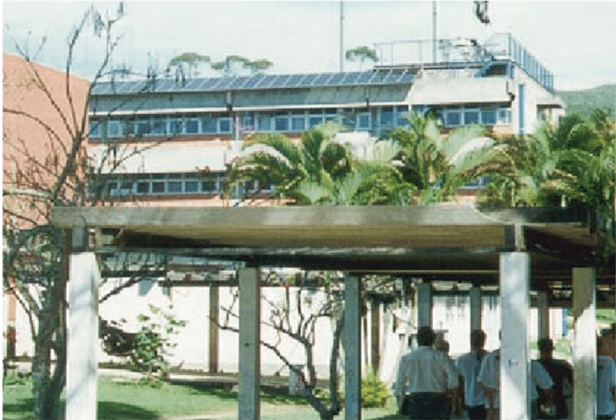
Fig. 18 The first grid-connected BIPV system in Brazil, installed on the LabSolar building in 1997 at the Federal University of Santa Catarina (UFSC) in Florianópolis, Brazil. This was one of several BAPV and BIPV systems pioneered at the university over the past two decades. (Source: Dr. Ricardo Rüther, UFSC, and Ref. [47])
