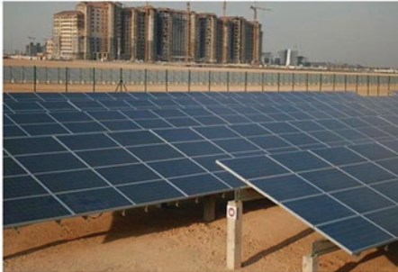
(b) Close up of the 87,780 solar PV power plant
