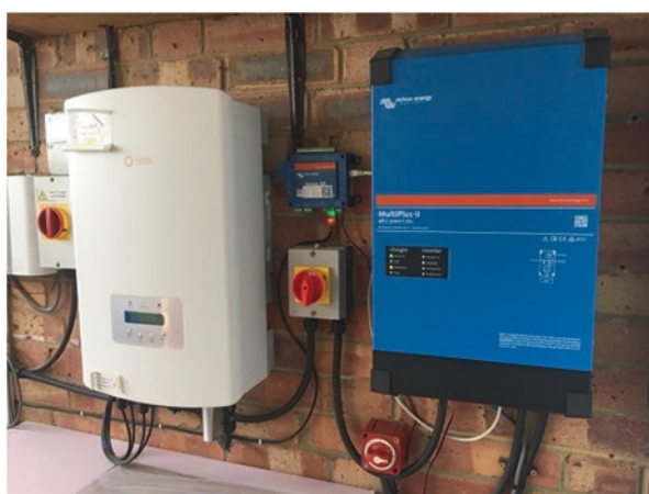
Fig. 14 Two inverters, on the left the PV inverter; on the right a charge inverter which controls the 10 kW battery system, which will be explained later
