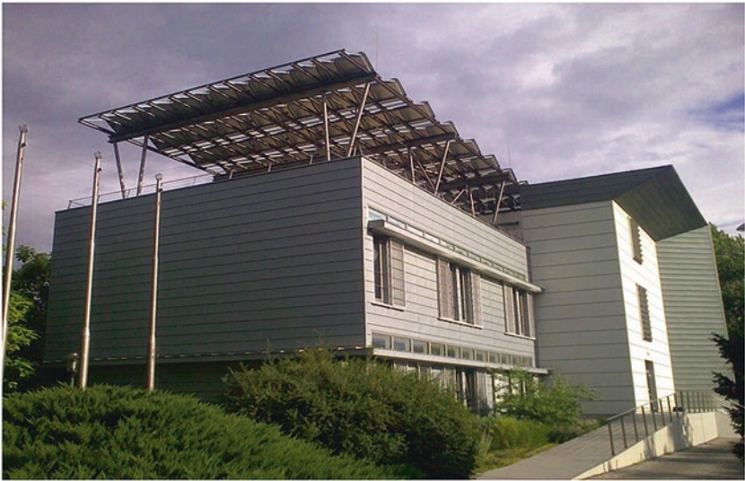
(b) Close up of the 29 kWp Solar PV array generating clean energy
