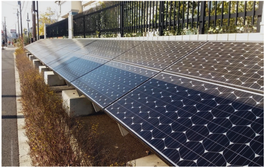
(b) The solar PV array, each generates 6 kW power output.
