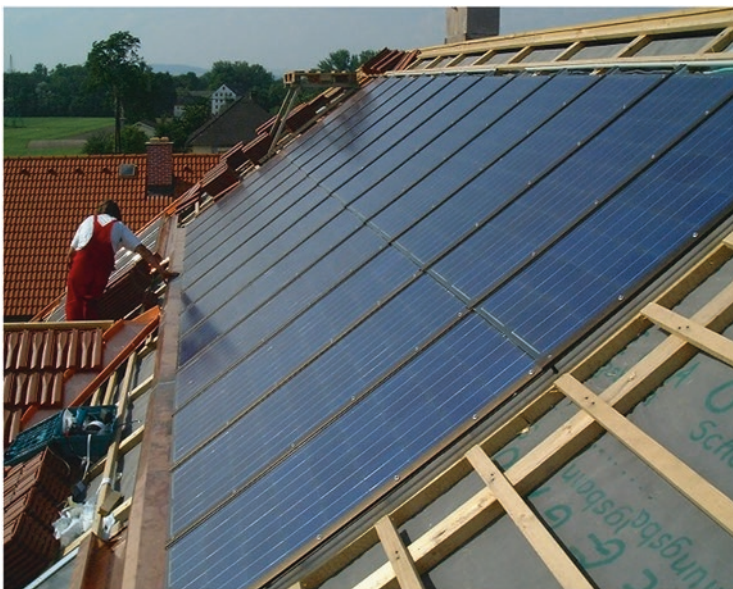
Fig. 5 Roof integration of the case study of a 3 kW-PV-system in Enns, Upper Austria
