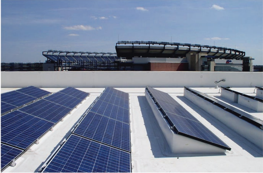
Fig. 14 Integrated solar photovoltaics panels on the roof of Gillette Stadium in Foxborough, Massachusetts in the USA. (Image credit and source: Chris Bills, Chris Erickson, Calla Leonard, and Patrina Eiffert, https://upload.wikimedia.org/wikipedia/commons/c/c1/Solar_cell_panels_on_roof_Gillette_Stadium_2010.jpg )
