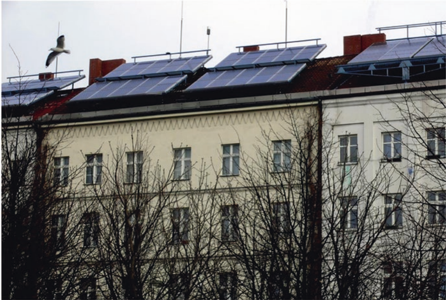
Fig. 16 Mounted Solar Photovoltaics' arrays on the rooftop of a block of buildings in Berlin, Germany. (Image source: https://upload.wikimedia.org/wikipedia/commons/4/45/Berlin_pv-system_block-103_20050309_p1010367.jpg )
