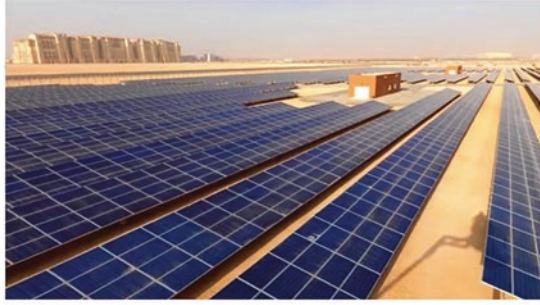
(a) The solar power PV plant in Master City
