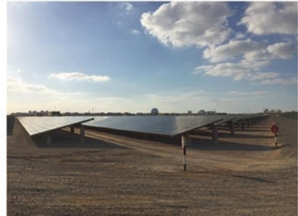
(c) View of two arrays of the PV plants
