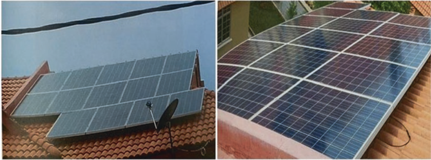
Fig. 22 7.8 kWp photovoltaic (PV) rooftop installation in a Malaysian home [59]
