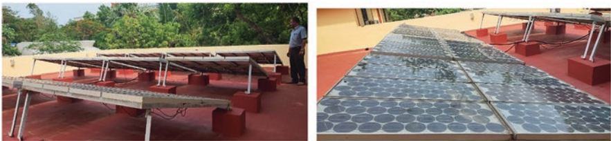
Fig. 12 CDD installation on the terrace
