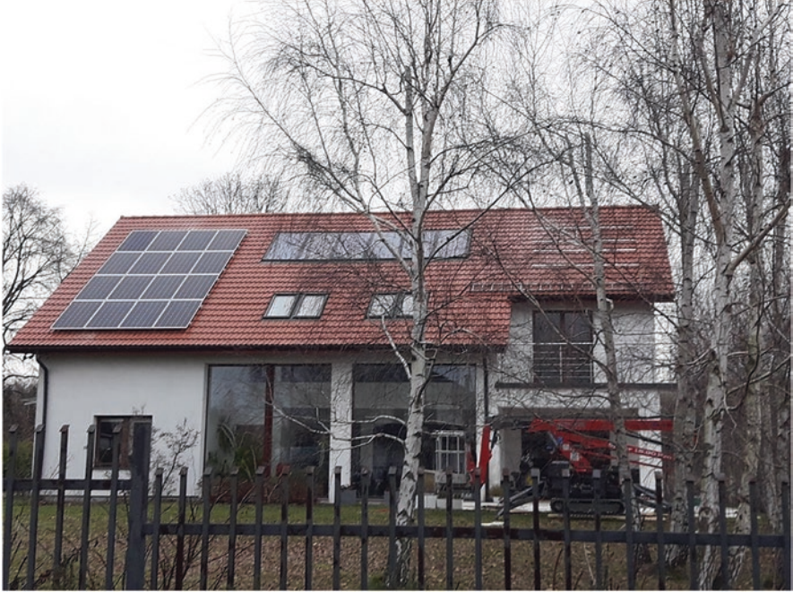
Fig. 8 Single-family house with BAPV system during its installation on the roof of the building
