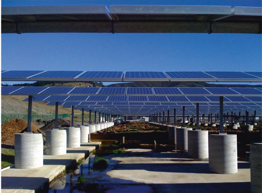
Fig. 18 Solar panels mounting system on the roof of Pacifica wastewater treatment plant in Pacifica, California, the U.S. (Image credit and source: Robert Scoble, https://www.wikiwand.com/en/Photovoltaic_mounting_system#Media/File:Photovoltaic_mounting_system.jpg )
