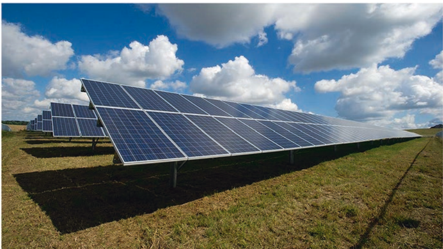
Fig. 2 Shotwick Park, solar farm, [5]
