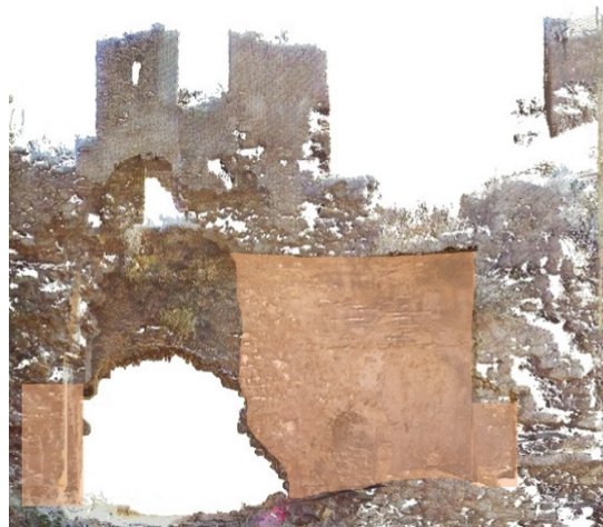
Fig. 8. Orthophoto from point cloud viewing the cross-section A-A with visibility to the interior of the Gate, including the Ottoman period construction phases (orange)
