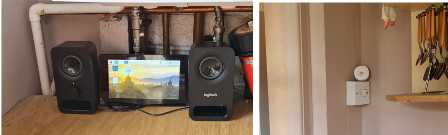
Fig. 1. IntraVox installed inside a cabinet (left) and the motion sensor (right).
