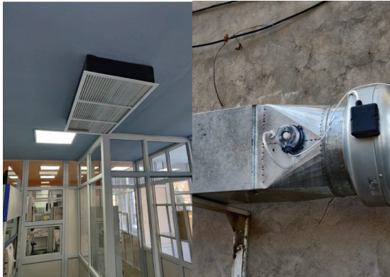
Fig. 6. Ventilation inlet for air quality control
