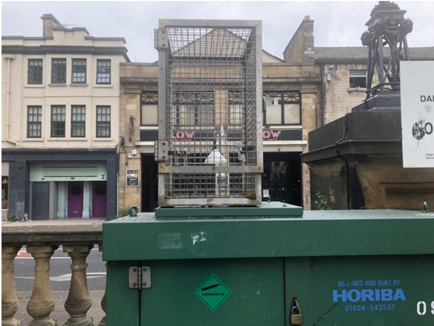
Fig. 6 Air quality monitoring device
