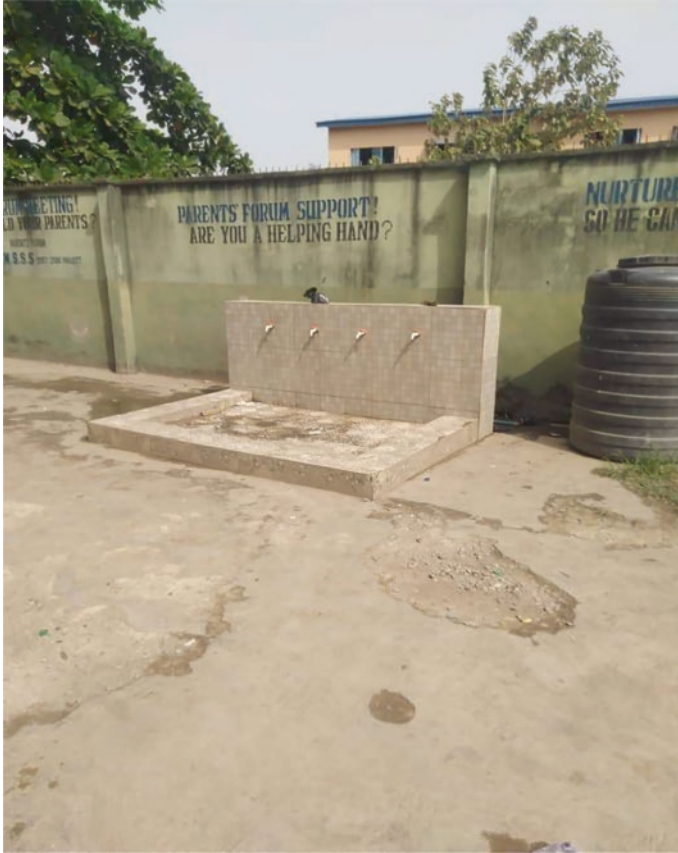
Fig. 14.4 Water Facility in one of the schools in Lagos state
