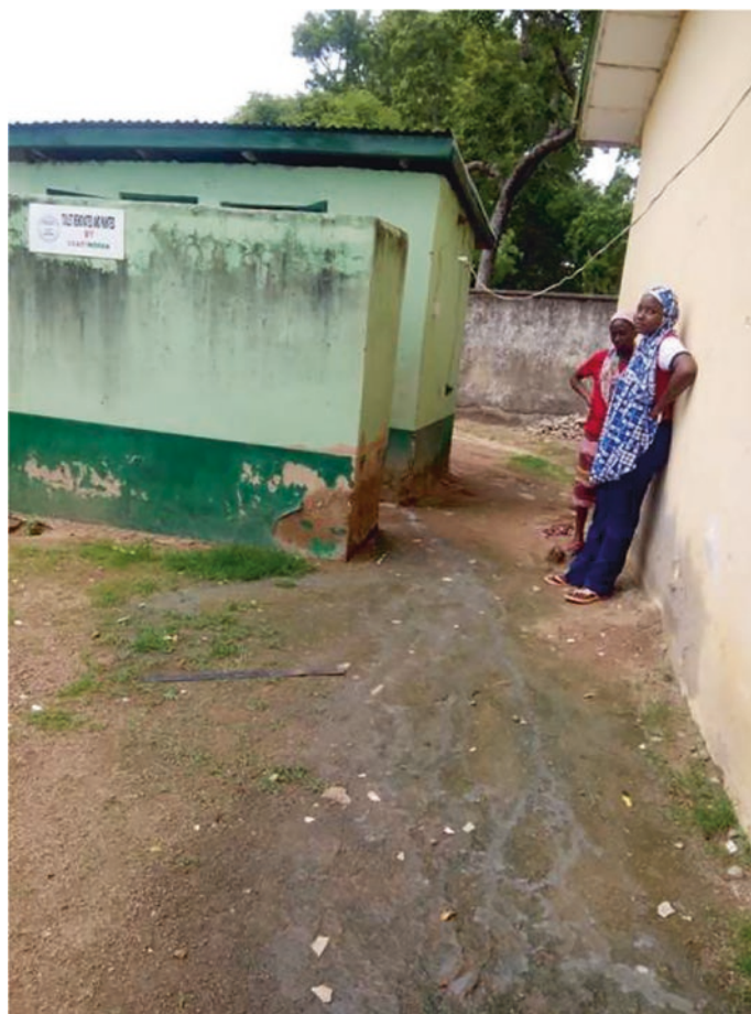
Fig. 14.7 Toilet facility in one of the schools in Bauchi state
