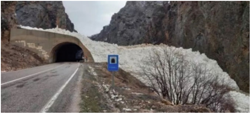
Fig. 11.10 A view of an avalanche on the Erzincan-Tunceli highway [66]
