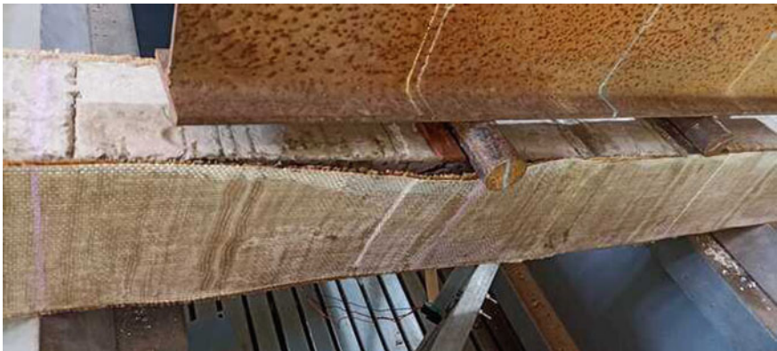
Fig. 9 Debonding of FRP from the surface of the beam
