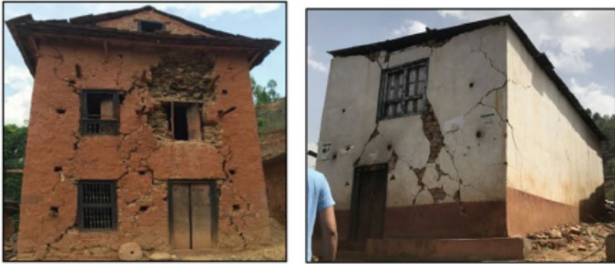
Fig. 1 Post-earthquake damage in masonry buildings in Nepal (Rohit et al.)
