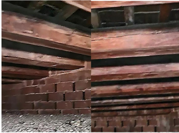
Fig. 3. Interior of the air chamber of one of the decks visited. Source: own elaboration.
