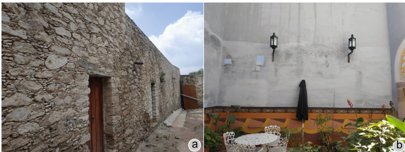
Fig. 3. View of the interested walls a) Northwest wall of Temple of Inmaculada Concepción b) Surrounding wall of Terán House
