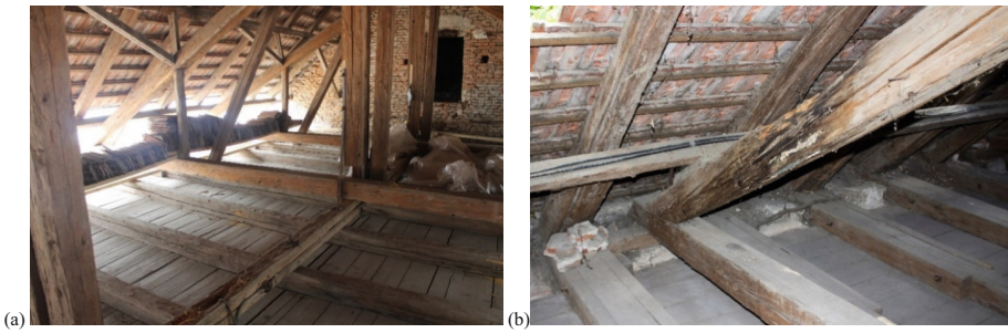
Fig. 4. Attic interior. Later interventions - longitudinal bracing elements and king post trusses (a). Biological decay (b)
