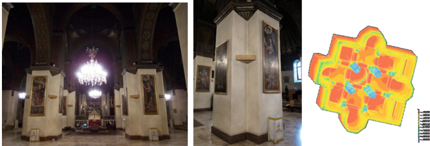
Fig. 14. Inside views and an estimated stress concentration for pillars (von Mises stress for D.L.)
