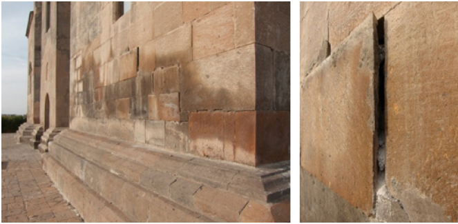
Fig. 8. Degradation of the outer wall in the southeastern corner
