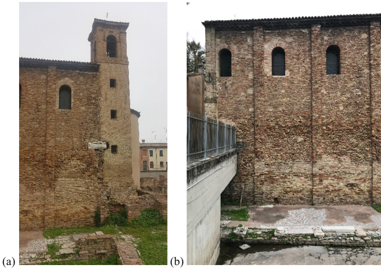
Fig. 12. Real damage pattern: (a) connection between the bell tower and the southern wall, (b) connection between the street and the southern wall.
