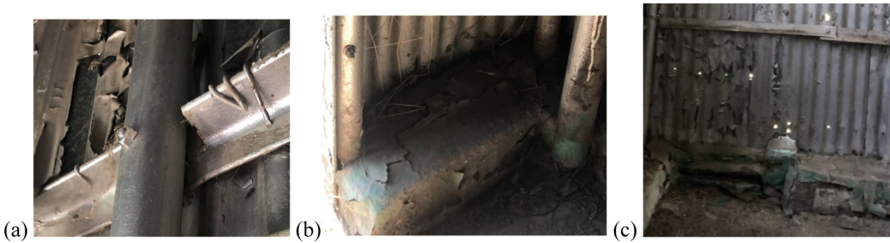
Fig. 6. a) Depicts the corrugated iron sheathing wall connected to both a pipe column and an angle beam using ties on an interior repetitive section, b) Depicts the concrete ledge in which a pipe beam is encased, c) Depicts corrosion that is seen throughout the sheathing.
