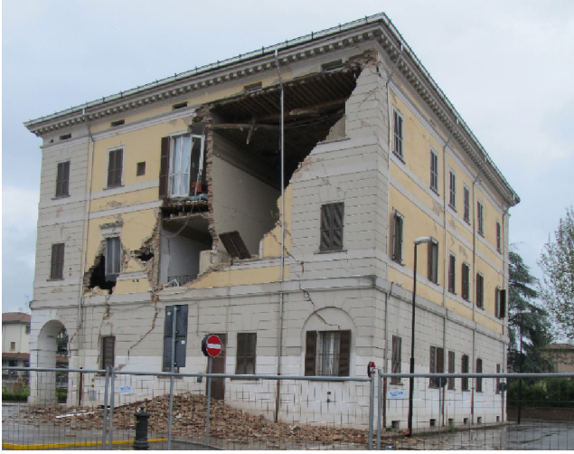
Fig. 1. Example of out-of-plane failure of URM wall connected to timber diaphragm during the 2012 Emilia, Italy earthquake.
