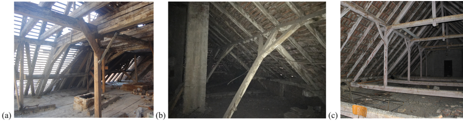
Fig. 1. Roof structures for the study - a) first roof structure; b) second roof structure; c) third roof structure [13]
