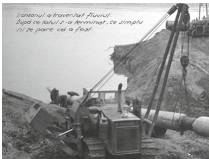
Fig. 7 The undercrossing of the Danube enabling gas imports from the former USSR (1979)
