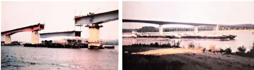
Fig. 13.97 Giurgieni-Vadul Oii bridge, views during construction (left) and in use, 1970 (right) (Buzuloiu 2006)
