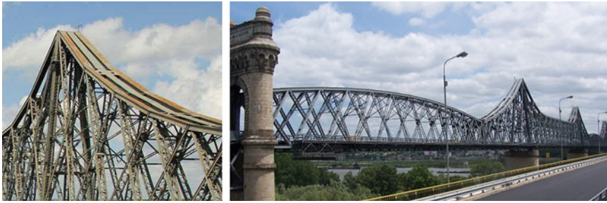
Fig. 13.96 Cernavodă bridge after strengthening, the detailed view with 3 chords for top chord (left) and overall view after strengthening (right) (Florea and Ionescu 2012)
