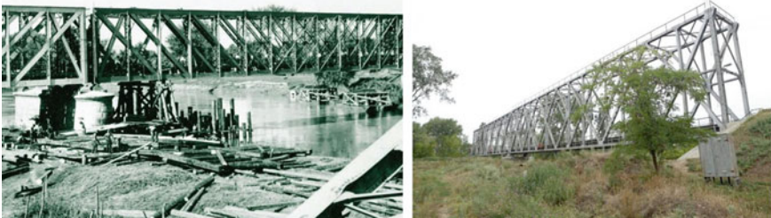
Fig. 13.40 The bridge over Prut River at Ungheni, under construction (left) and today (right) (Popescu 2014)
