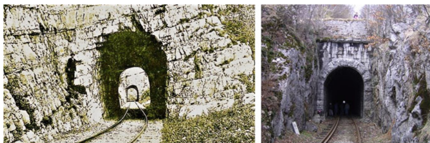
Fig. 13.44 Tunnels without waterproofing on the lines Oravița–Anina (left) and entrance portal in the tunnel Gârlișteța (right) (Popescu 2023b)
