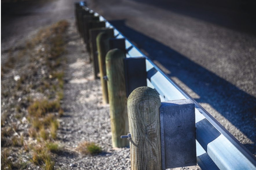
Fig. 3.15 Guardrails on bridges should not be crossed
