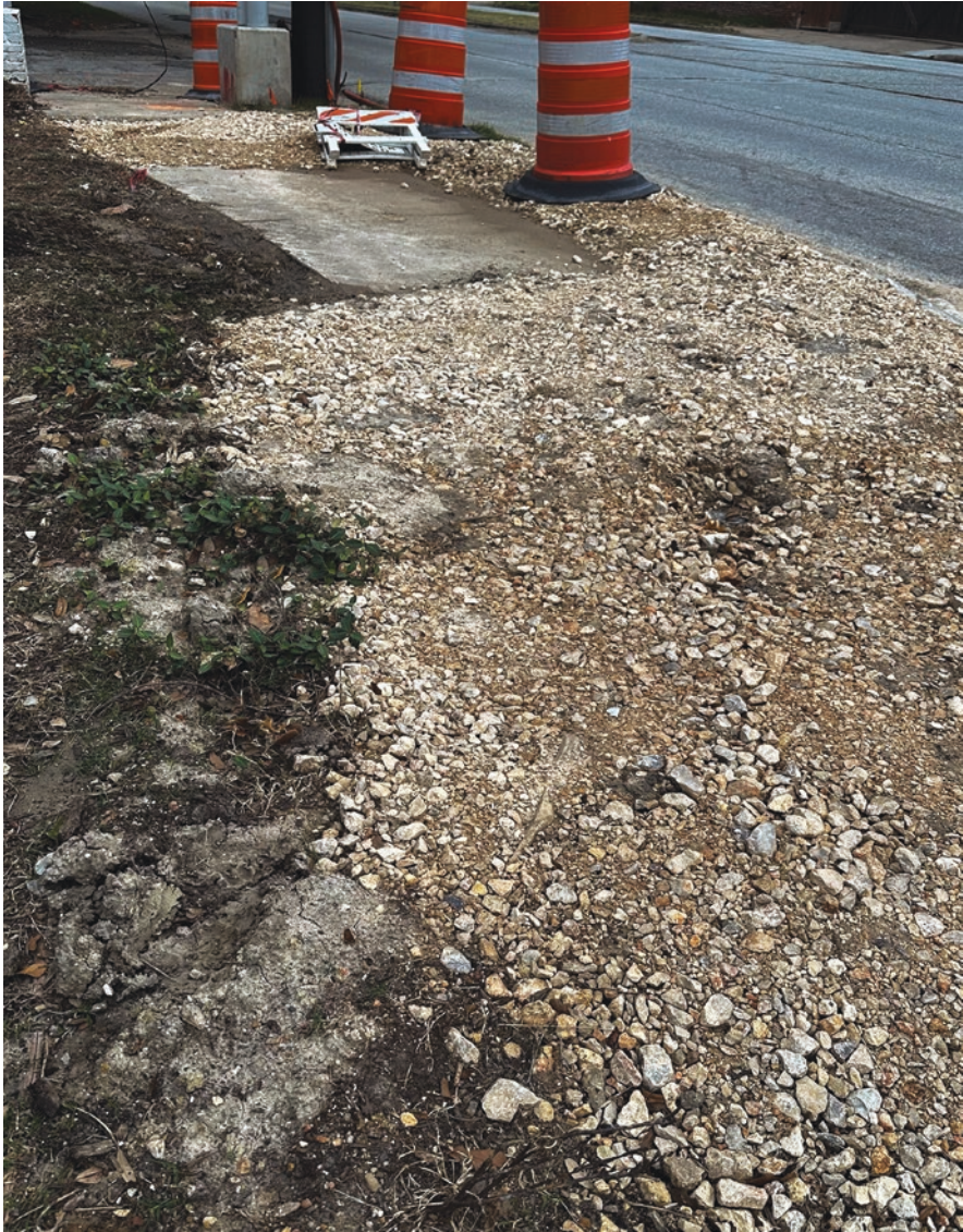
Fig. 3.5 It is easy to trip over an uneven surface. Those with impairments should use caution
