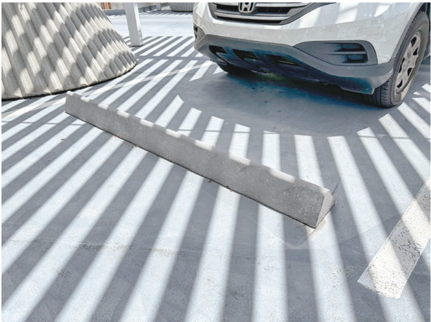
Fig. 6.6 It is easy to trip over uneven surfaces or parking blocks. Those with impairments should use caution and be aware of this potential hazard
